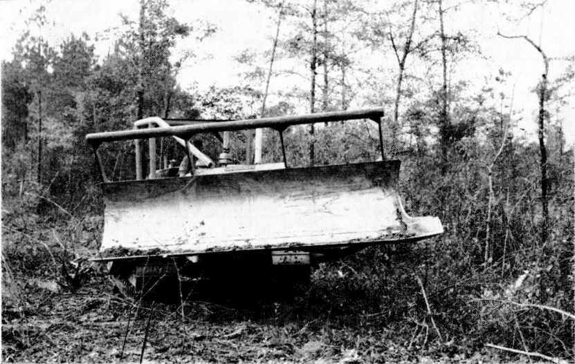
FIGURE 2. (Above) Bulldozer blade mounted on crawler-type tractor used in the experiment. Note holes left after removal of stumps with dozer blade. (Below) Mounted KG blade used in land clearing test.
