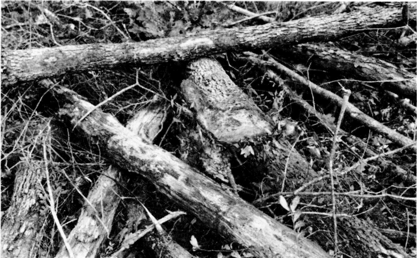
FIGURE 3. Trees sheared off and felled with the KG blade mounted on tractor.
