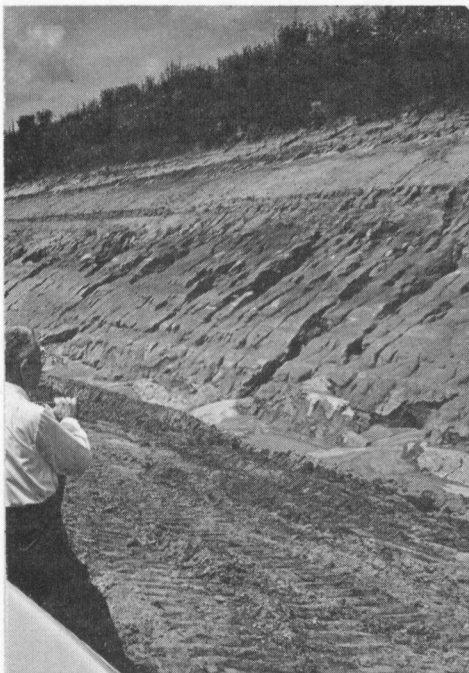
This is typical erosion damage from washing rains on unprotected back slopes.
