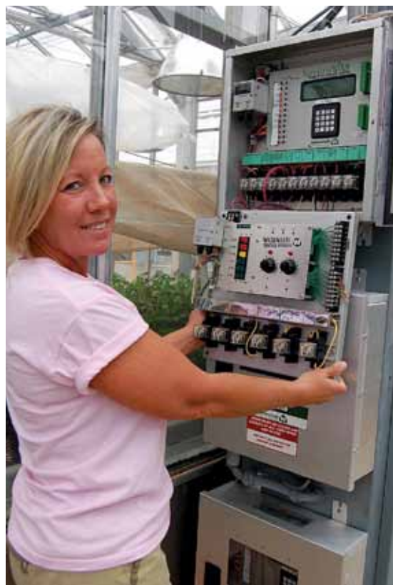
OUT WITH THE OLD —Jane Hoehaver Farr holds one of the old Wadsworth greenhouse climate controls installed when the Plant Science Research Center was built in 1991 beneath one of 12 new, advanced and digital Wadsworth EnviroSTEP climate controls that now manage and log the temperature, humidity and more in each of the PSRC greenhouses' 12 zones.
