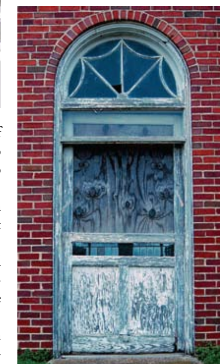
RETAINING PAST BEAUTY —Design ideas put forward by the Design-Build student team incorporated the dairy barn's unique elements, such as this lovely window, into the new plan, thus retaining the building's historical integrity while showcasing its architectural beauty.
