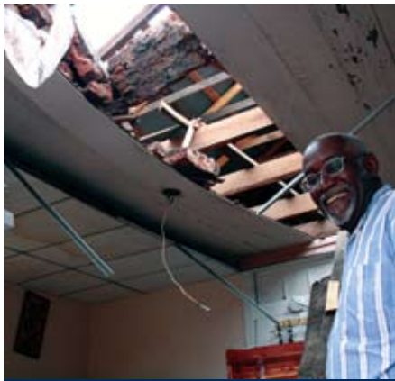
SKYLIGHTS THE HARD WAY —Thanks to a tornado packing 150-mile-per-hour winds, Curtis Jolly's house now has several rooms open to the sky. The roof and ceiling of this room, where Jolly was standing when he first heard a frog's frantic warning, partially blew away and partially collapsed inward, chimney and all.
