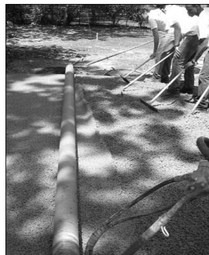
PAVING THE WAY —Auburn building science and biosystem engineering students smooth freshly poured pervious concrete in the arboretum parking lot in April.
