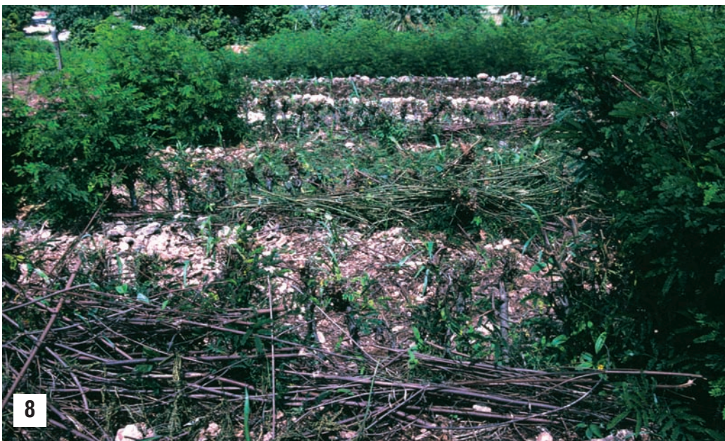
Photo 8. Branches are placed at the base of the hedgerows on the uphill side in order to reinforce the barrier. Pernier, Haiti.
