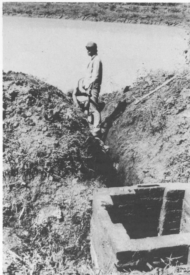
Water supply conduit system construction at the Fish Culture Center at Atiocoyo, La Libertad.
