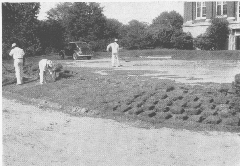
Sodding an area solid with blocks of Bermuda grass sod. On the right, are the blocks of sod, while at the left the area has been sodded solid by putting the blocks in place.
