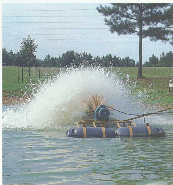
FIG. 2. A 10-horsepower electric pond aerator in operation.
