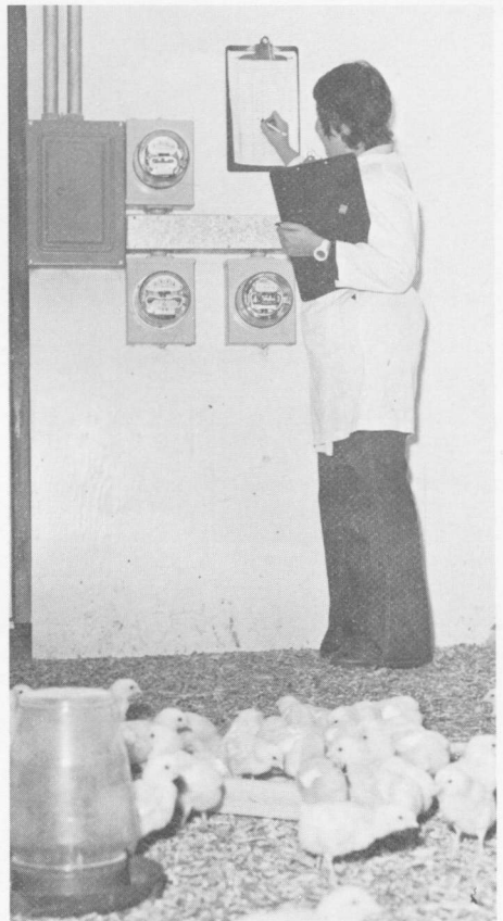
Sub-metering of circuits for fans, lighting, and outlets in each pen provides data on energy use in test pens.
